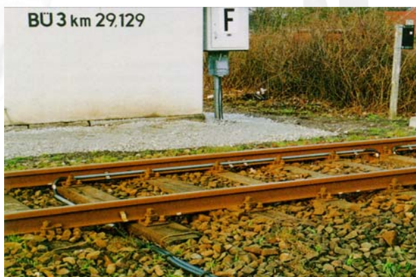
installed induction loop
